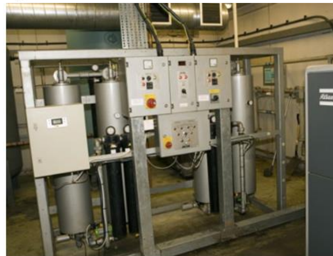
Fig 2 Medical air compressor
