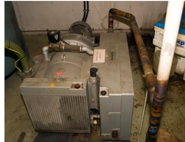
Fig 4 Suction is generated by a large vacuum plant within the hospital
