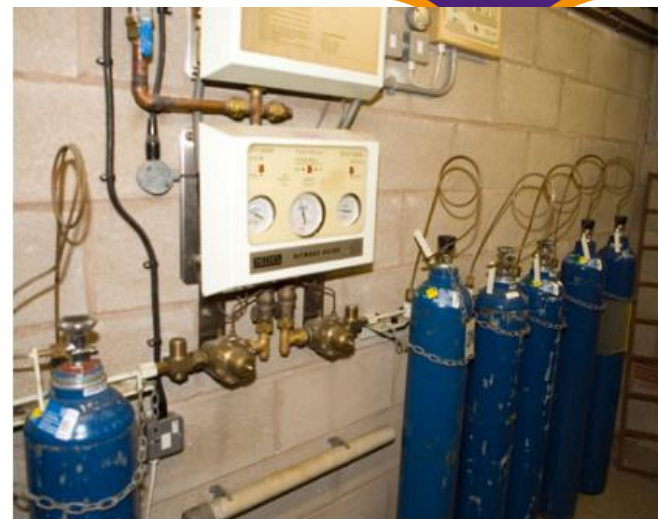
Fig 1 Nitrous oxide bank or manifold
