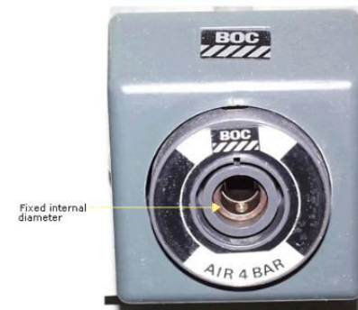
Fig 5 MA4 outlet showing fixed internal diameter
